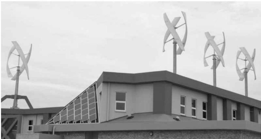
Figure 10: Vertical axis generators in conjunction with photovoltaic seen in Swakopmund Photo: Amusha (2015).
